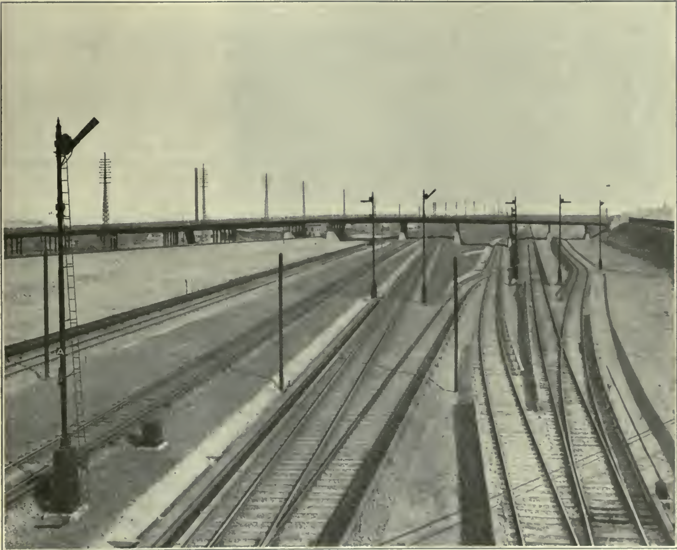
FIG. 505. THIRD RAIL CONTACT SYSTEMS. Main Track Construction, 600-Volt Over Running Third Rail Installation, Pennsylvania Railroad, New York City.
